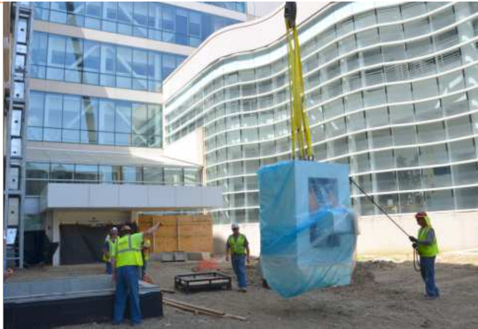
Cyclotron installation at the Bill and Rita Clements Advanced Medical Imaging Building
