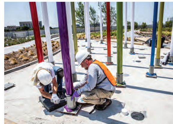
Poles were bolted to the rooftop floor, then the bases were covered in gravel.
