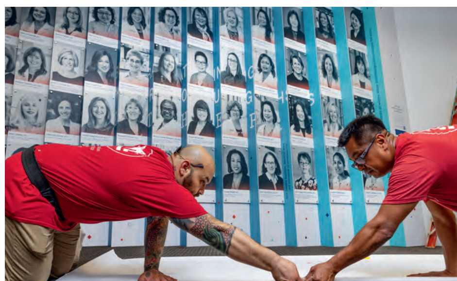
Workers with Mecca, subcontractors to designing agency Johnson & Sekin, complete the installation.
